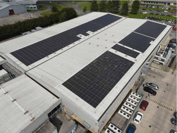
Waterton office solar panel — UK
